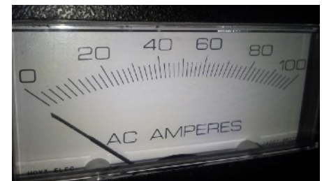
Amp Gauge (power using)
